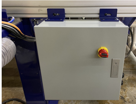
Figure 2: Close-up of mounted control box.
